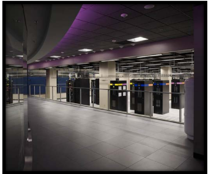
Cerner WHQ location servers and data center.
